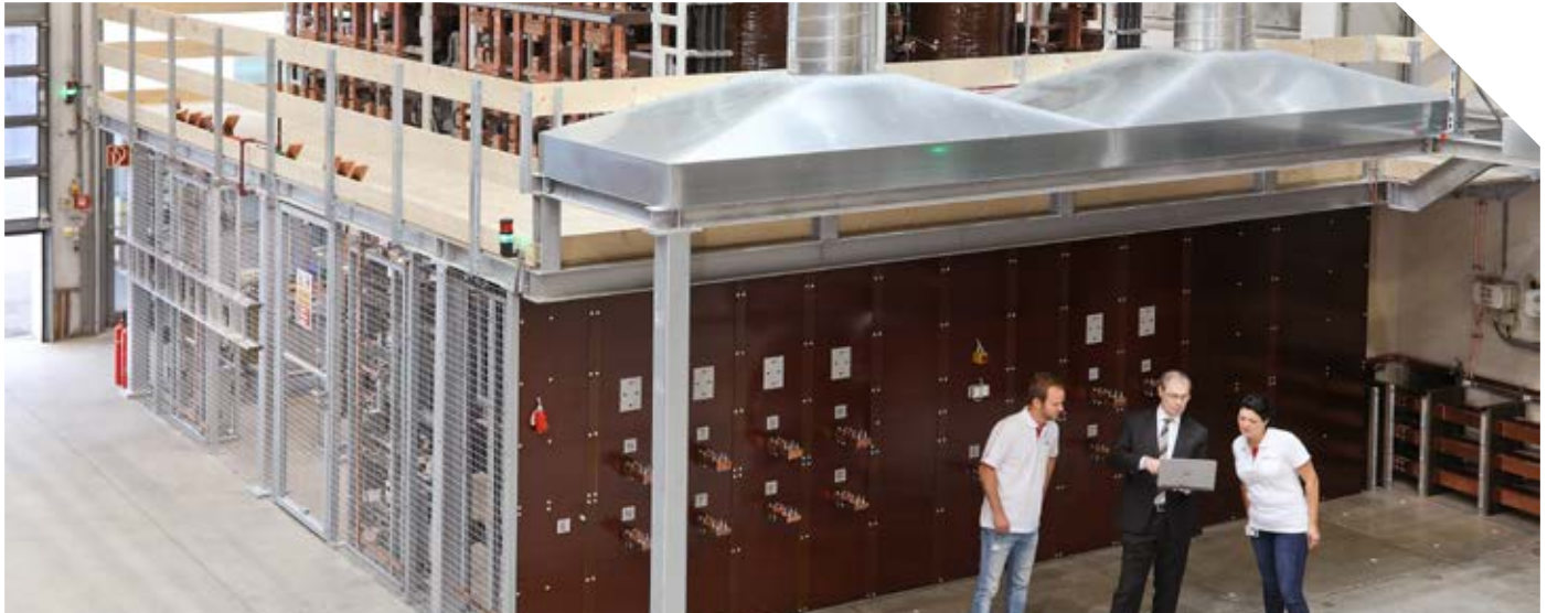
The AIT DC Lab offers companies a state-of-the-art platform for the development, testing, and validation of DC components.
